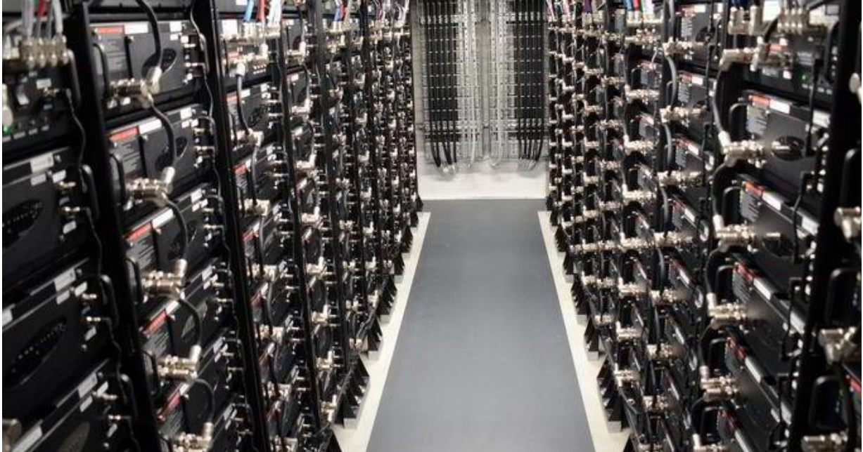
Battery system. Source: https://www.europower-energi.no .
