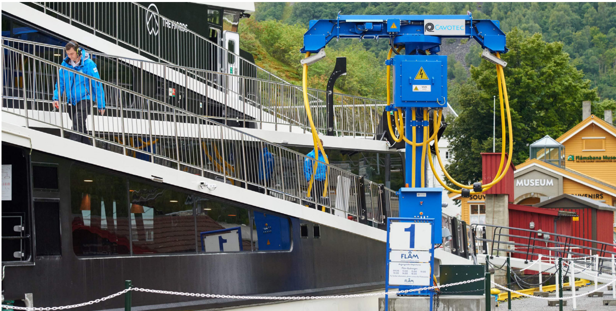
Remotely-controlled land-based electricity connection at the quayside in Flåm. Image: CAVOTEC.
